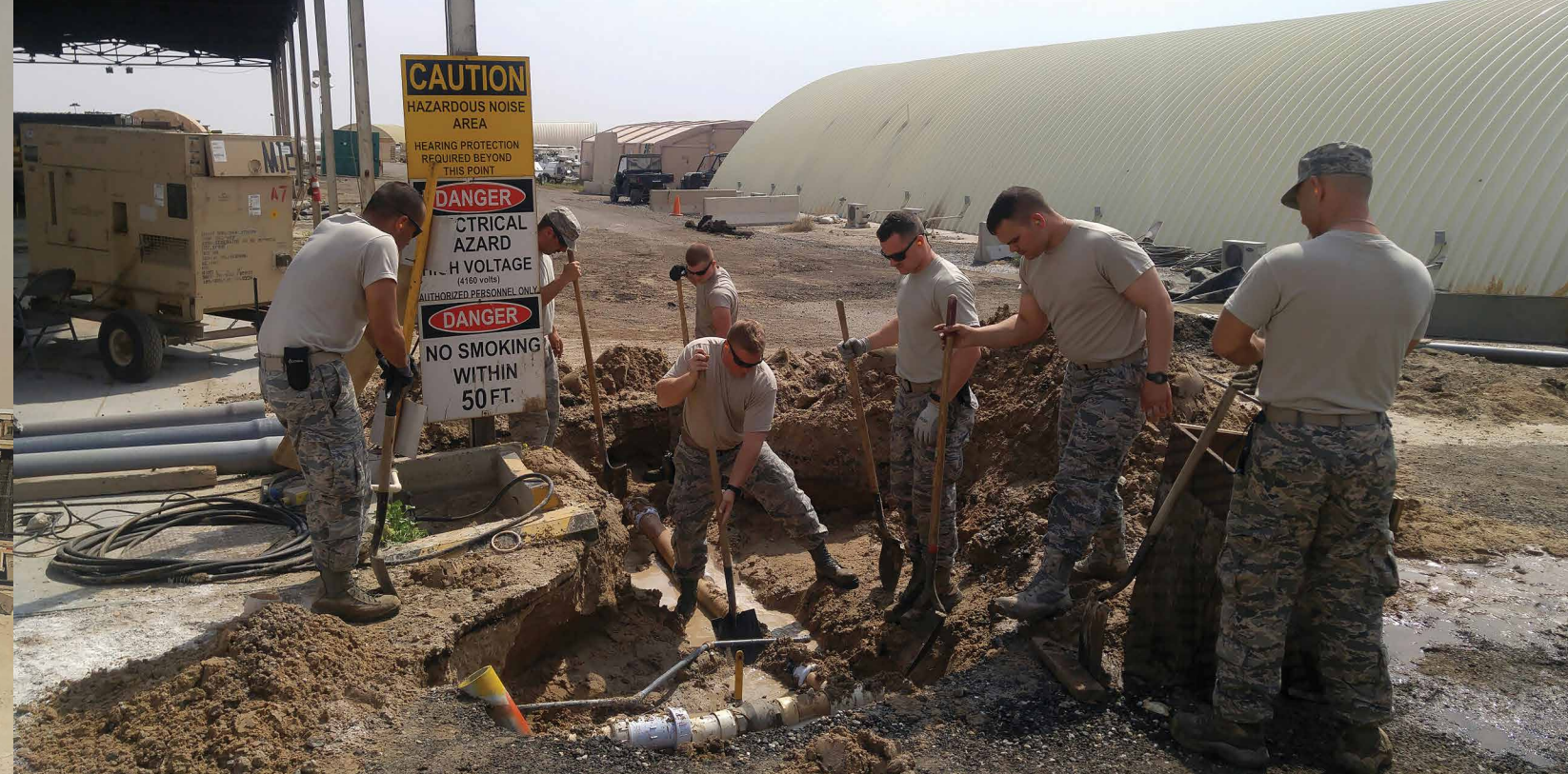
Engineers work in the heat of Southwest Asia to finish installation of much-needed fuel and control lines. (U.S. Air Force photo by Tech. Sgt. Donald Jabaay)
