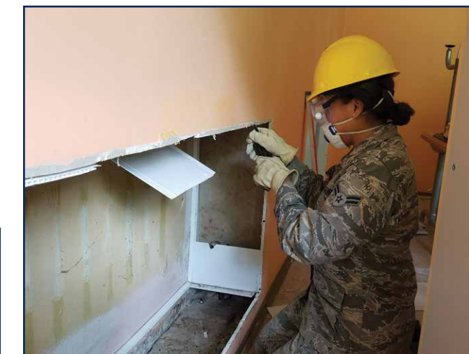
Airman 1st Class Angeles Cruz-Morales cuts to fit a section of wall in preparation for new drywall installation. (U.S. Air Force photo by Staff Sgt. Nicholas Goldman)
