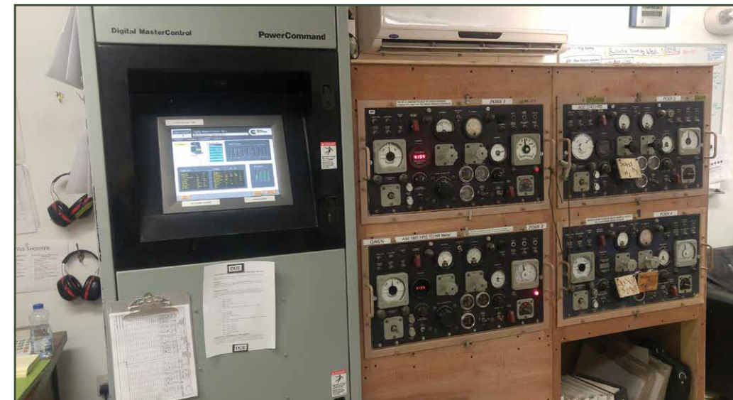
Different technologies were used on site to include the digital interim base expeditionary airfield resources and analog MEP-12. (U.S. Air Force photo by Tech. Sgt. Donald Jabaay)
