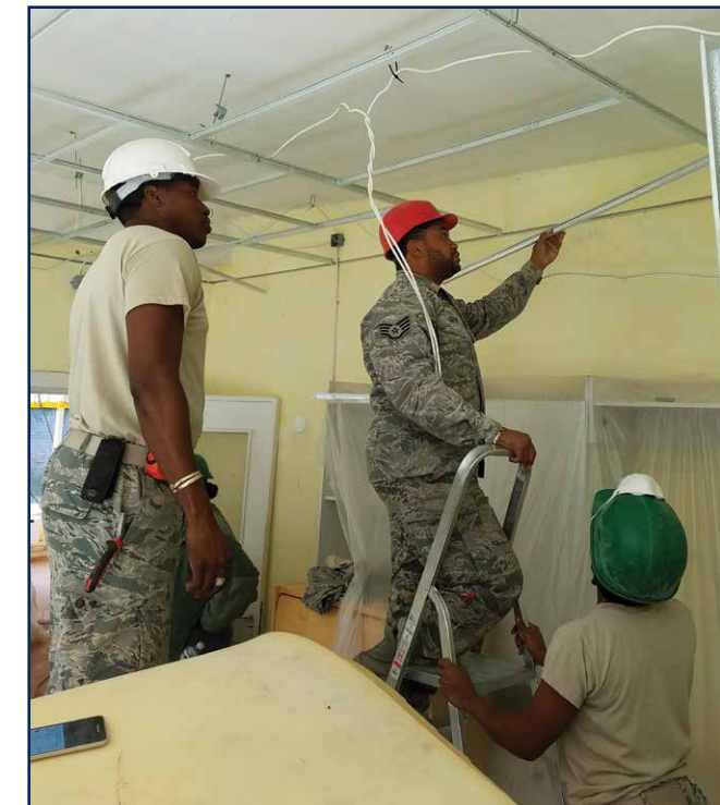
From left, Staff Sgt. Anthony Harley, Staff Sgt. Jamale Griffin and Senior Airman Vanessa Ayala of the 285th Civil Engineer Squadron structural team install a drop ceiling. (U.S. Air Force photo by Staff Sgt. Nicholas Goldman)
